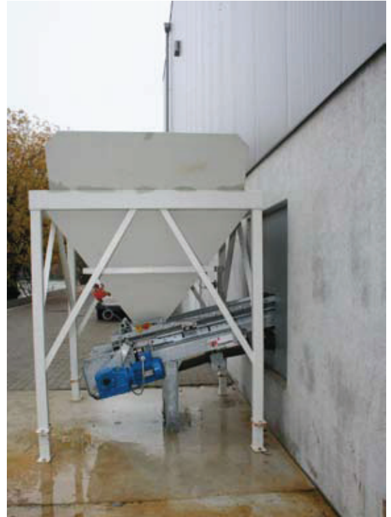
Fig. 5 The production hopper for special aggregates: big bag discharge through outside hoppers and dosing conveyor possible.
