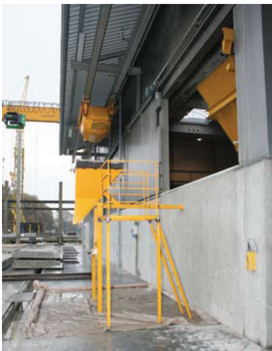
Fig. 1 The silo is fed via the outside bucket conveyor supplied by company WMW.
