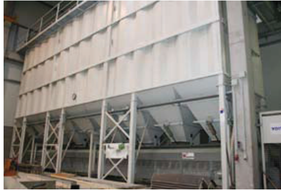
Fig. 3 The row-type silo plant with dosing flaps and weighing conveyor at the head end of the production building.
