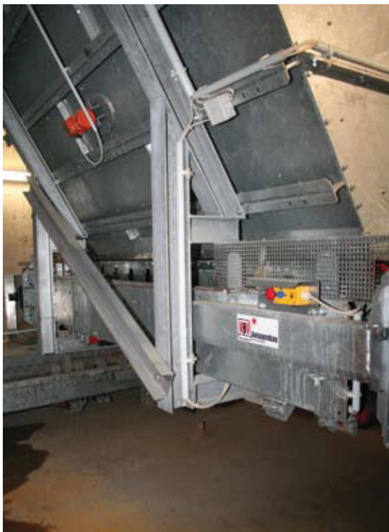
Fig. 6 Inside the feeding bunker where the aggregates are transported to the double belt conveyor by the transverse conveyor belt: material bunker for 20 m 3 of gravel with discharge conveyor.
