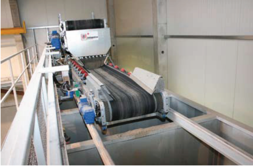
Fig. 8 In this way, the raw materials are carried from the double belt conveyor into the single silos. Abb. 8 So gelangen die Rohstoffe vom Doppelgurtförderer in die einzelnen Silos.
